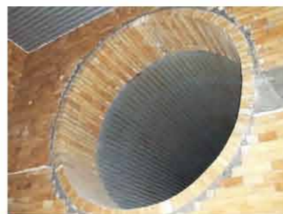
● 鋼鐵廠蓄熱塔施工 Construction of the heat accumulation Tower of Steel plant.
