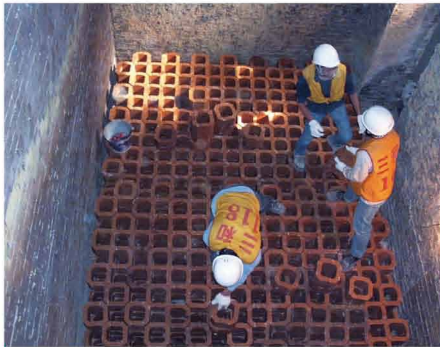
● 玻璃窯爐蓄熱室磚施工 Construction of the regenerator of glass furnace.
