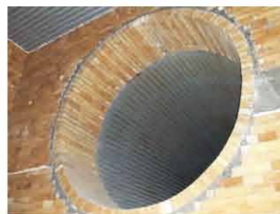
● 鋼鐵廠蓄熱塔施工 Construction of the heat accumulation Tower of Steel plant.
